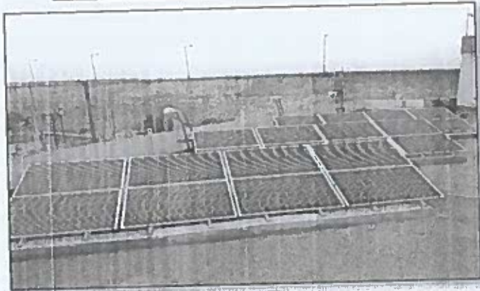
Solar PV Plant in Ash Pond.
