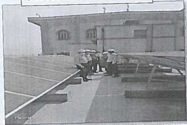
Solar PV Plant in Service building
